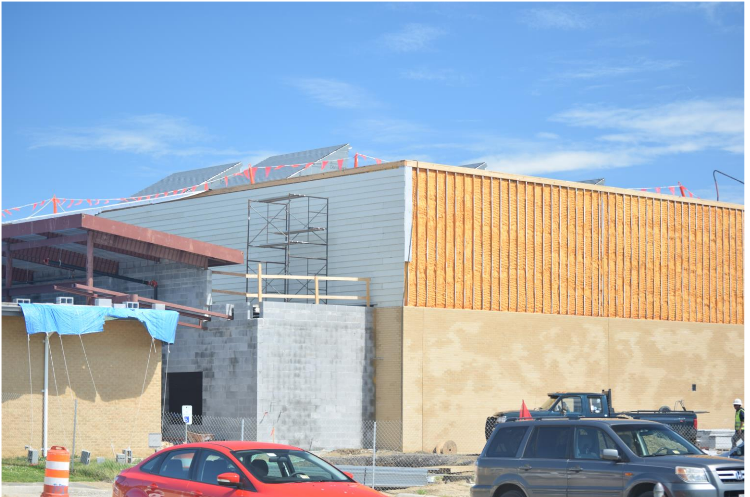
Work continues on modernizing John B. Dey Elementary school. For details on the project, click here: http://www.vbschools.com/school_renovation/schools/JohnBDeyES.asp
